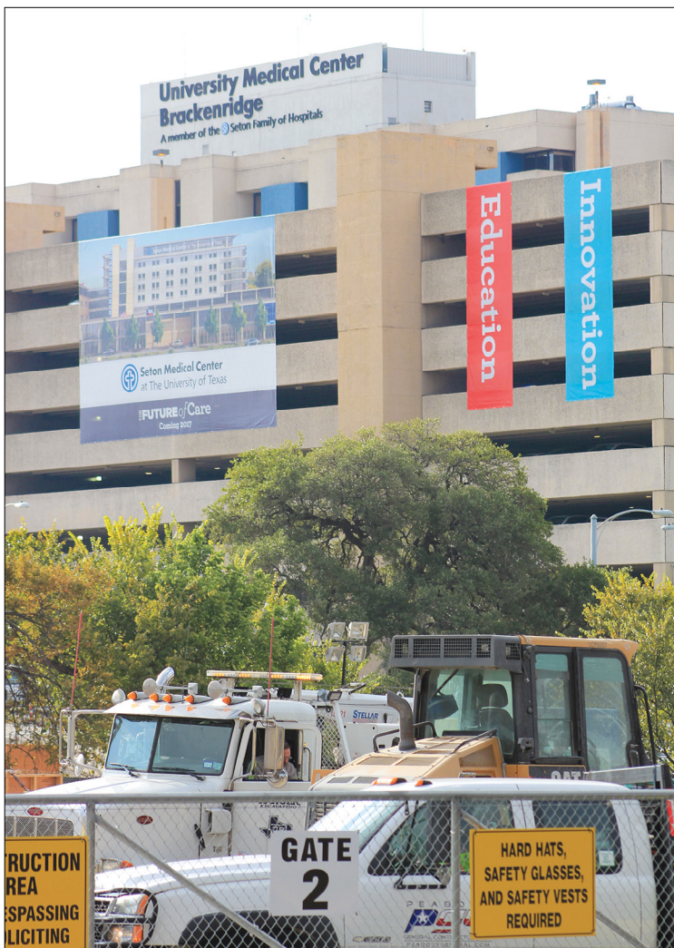
Construction in progress on the Seton Medical Center at The University of Texas at Austin. Photo courtesy of Ginger Lowry
