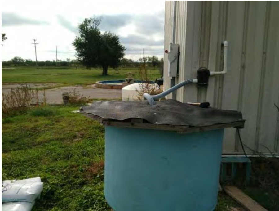
Figure 17. A chlorinated sand filter system at The Uvalde National Fish Hatchery Quarantine Building. Photo credit: USFWS.
